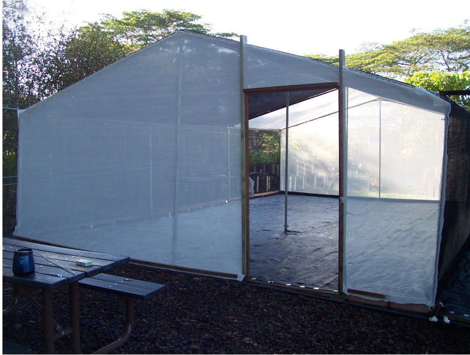
Figure 1.18. The new ANRPO shade house at their East Base Facility from 2005. As of 1/23/24, the EZ up poles are still standing but have a significant amount of rust, making this setup ideal for short term applications. Note the original weed mat flooring which was eventually removed in favor of gravel after ~10 years.
