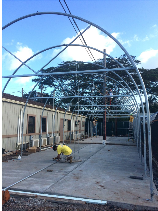
Figure 1.17. Newly poured concrete floors in ANRPO’s Skeeteretum. Note the overhead communication lines and telephone pole between the two structures (not ideal).
